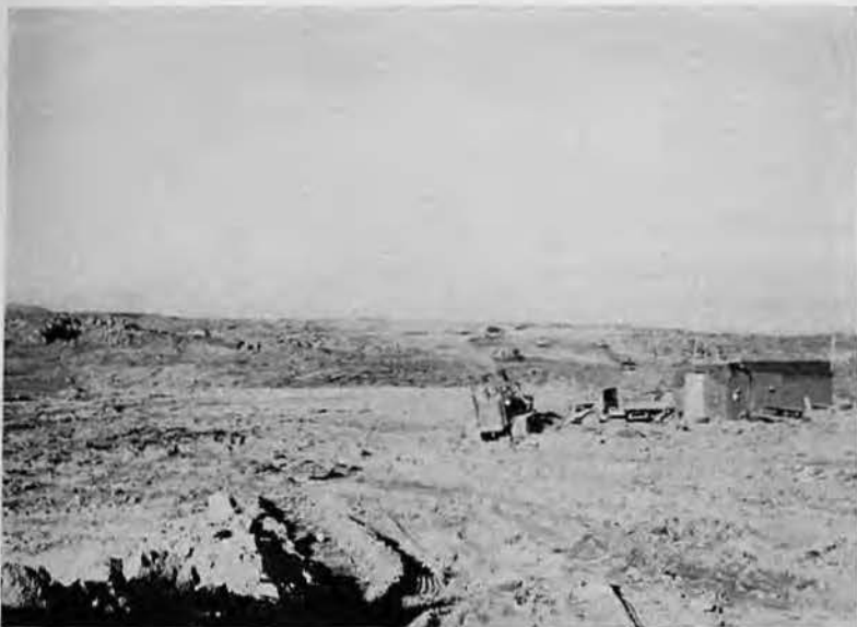
Portable Job Office and Lighting System Moved to Scene of Airstrip Extension.
